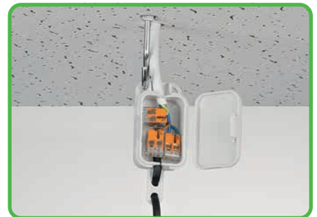
Pendant light connection in suspended ceilings
